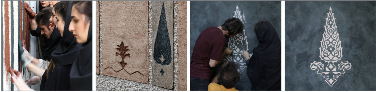
Figure 4. Lime plastering and Sgraffito of wall in 2 layers. The final layer of plaster should get scratched back before it sets too hard.
